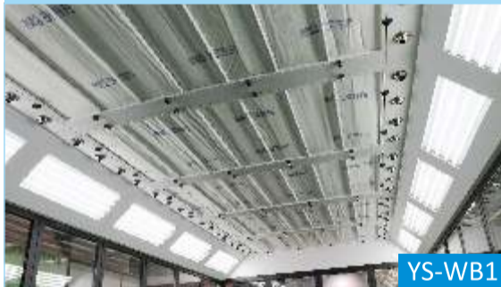
Waterborne Paint Drying System
